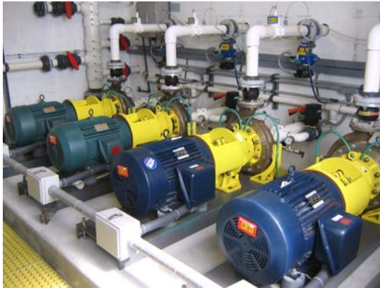
Main Pump Room
