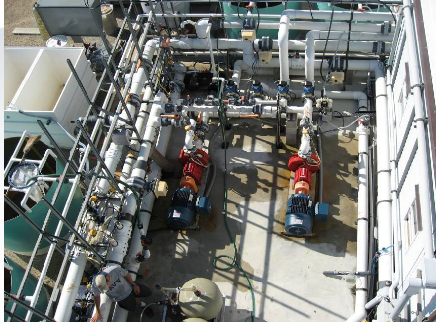
Ballast Pump, Sampling & Injection Skid
