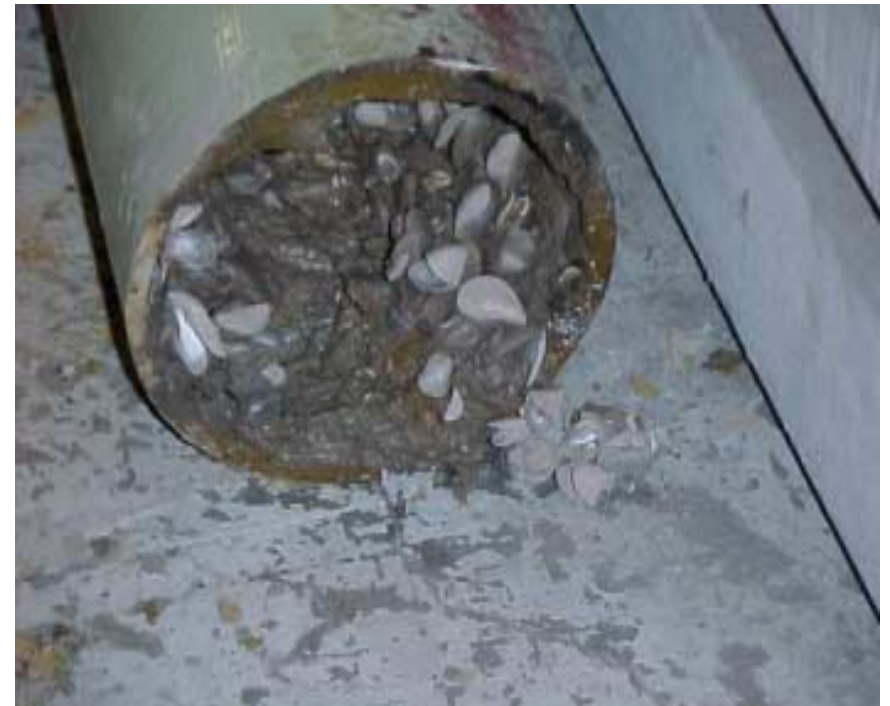
Water Cooled Transformer Piping at DeCew in 1999
